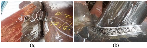
Figure 1 Complex joints of the jack-up legs: (a) joint before welding, and (b) joint after welding.
